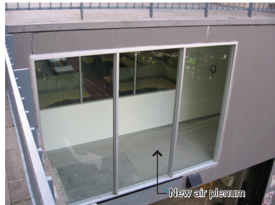
Figure 10. New window and air plenum The existing air grille was removed and the aperture glazed, with an additional glazed panel added to the internal partition. This allowed daylight to enter the room beyond, and the space between the walls to act as a plenum.
