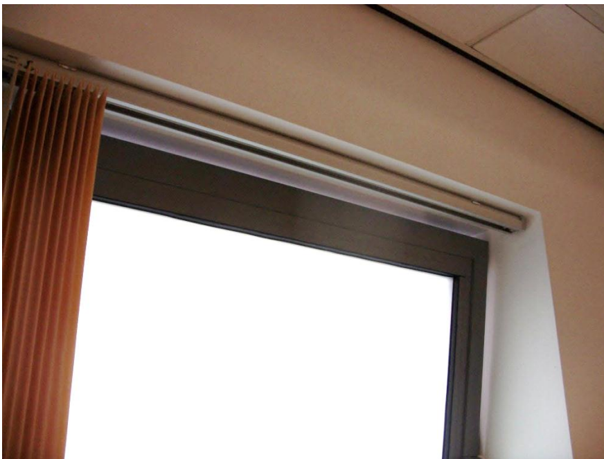
Fig 1 How not to integrate blinds and open windows
