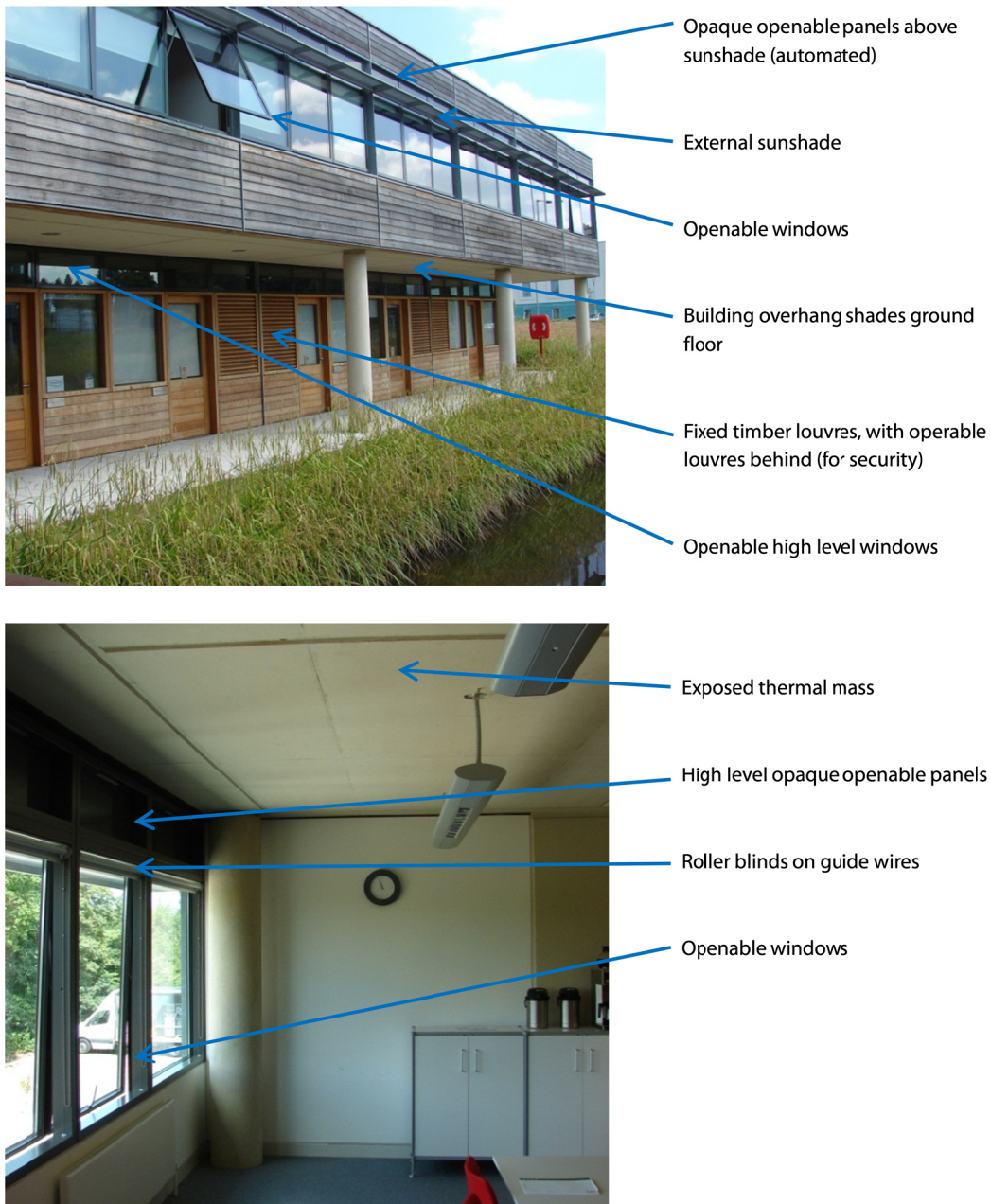
Fig H.21 Natural ventilation strategies at Butterfield Innovation Centre, Luton (photos: author)
