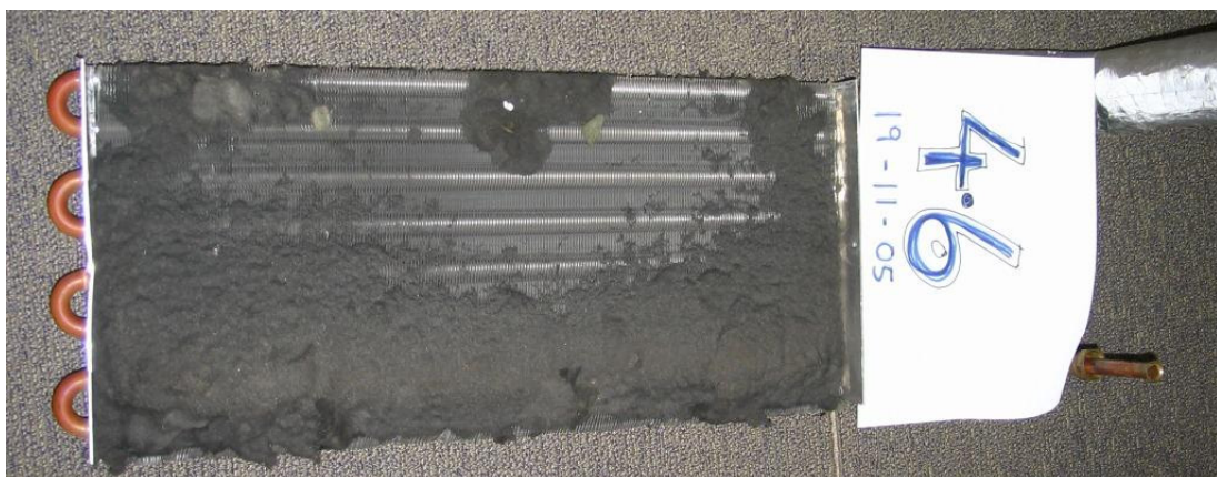
Fig H.23 A not so clean VAV heating coil
