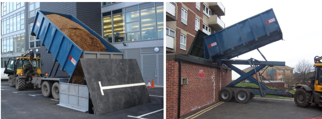
Fig I.9 Wood chips being delivered by trailer (photos: Eenergy - a British Gas Company [left], Dick Bradford [right])
