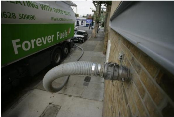
Fig I.8 Wood pellets being pumped into a building (photo: Forever Fuels)
